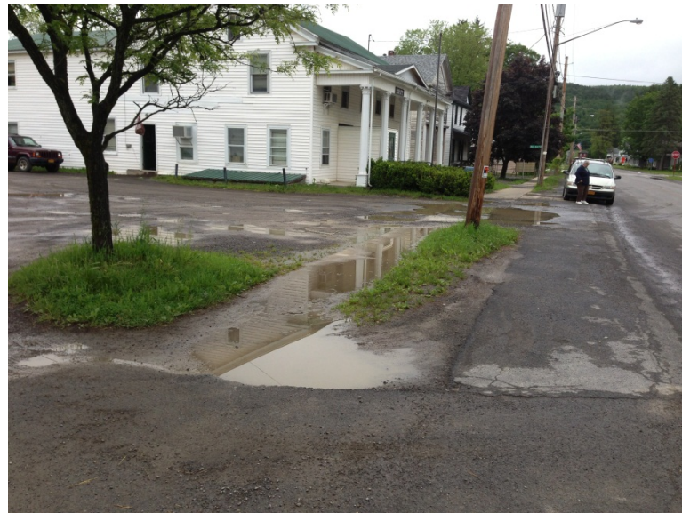
Figure 5: Main Street after county reconstruction. Notice the water pooling on sidewalks, inadequate parking strip, and generally ugly appearance.
