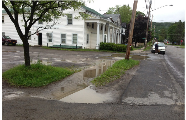
Figure 4-5: Main Street after county reconstruction. Notice the water pooling on sidewalks, inadequate parking strip, and generally ugly appearance.
